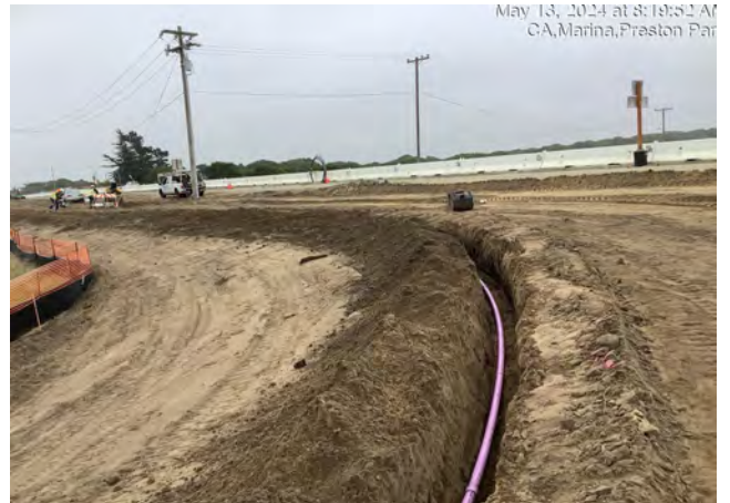
Irrigation service line at Preston Drive
