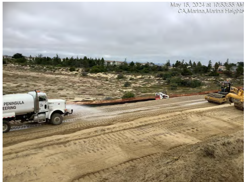
Dirt from south (eastbound) side of Imjin Parkway being moistened and compacted in fill on north (westbound) side of Imjin Parkway
