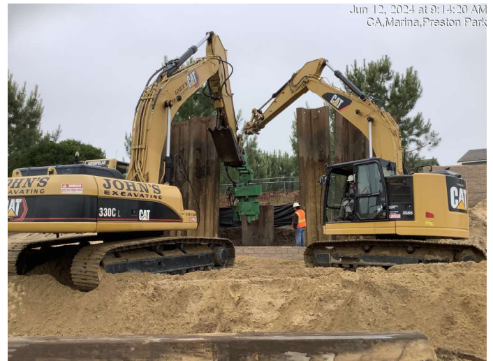
Removing temporary sheet pile shoring at retaining wall between Preston Dr. & Abrams Dr.
