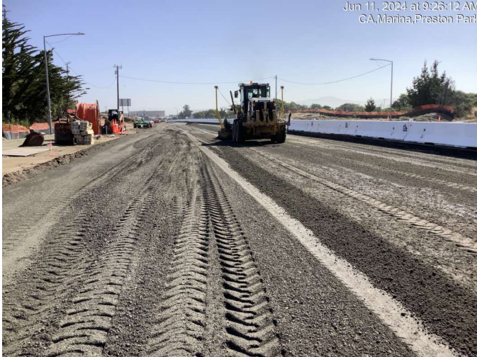
Installing & grading base rock material for subgrade of new roadway section between Preston Dr. and Abrams Dr.
