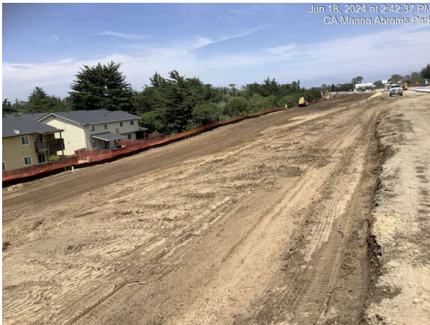
Earthwork operations for fill slope between Abrams Drive and Marina Heights Drive
