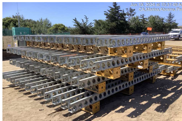
Materials for form panels to construct concrete retaining wall near Abrams Drive
