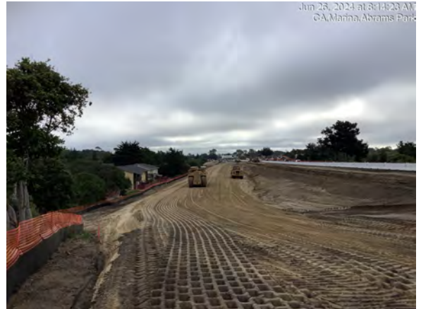
Equipment spreading and compacting dirt at fill slope between Abrams Drive and Marina Heights Drive
