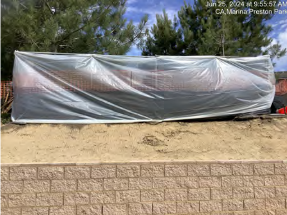
Plastic sheeting to protect sensitive plants (behind fencing) from any anti-graffiti coating over-spray
