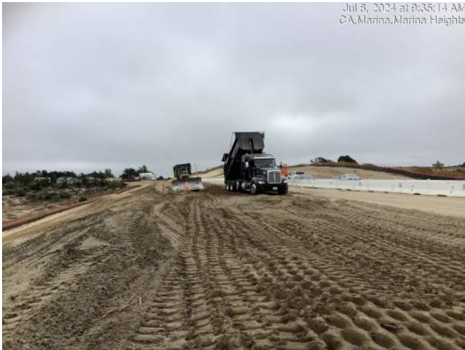
Earthwork operations for construction of fill slope between Abrams Drive and Marina Heights Drive
