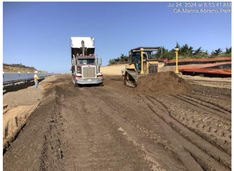
Imported soil material being graded to construct fill slopes between Abrams Drive and Marina Heights Drive
