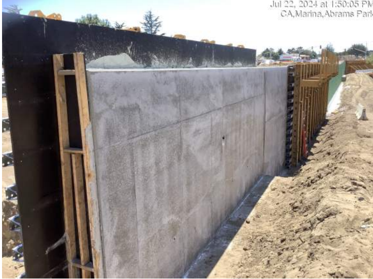
Forms are removed and curing compound is applied to the wall surfaces to retain moisture while the concrete cures.
