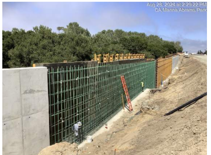
Forming for another section of the concrete retaining wall near Abrams Drive
