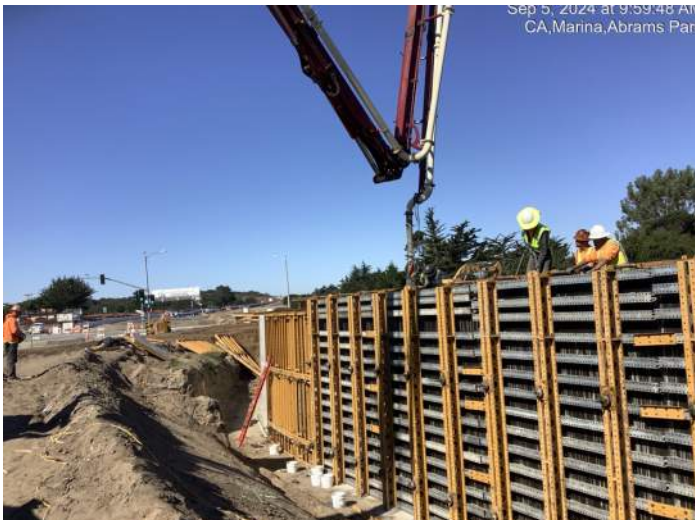
Concrete placement for final sections of the concrete retaining wall near Abrams Drive
