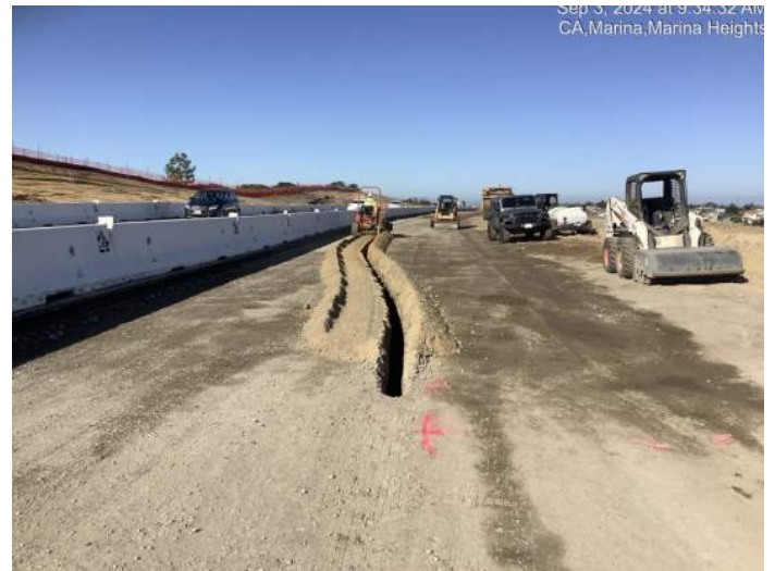
Trenching for street light & fiber optic conduits in future median area between Abrams Drive & Marina Heights Drive
