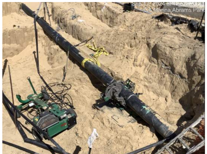
Fusion welding machine making one of two final tie-in welds for Army's treated groundwater system
