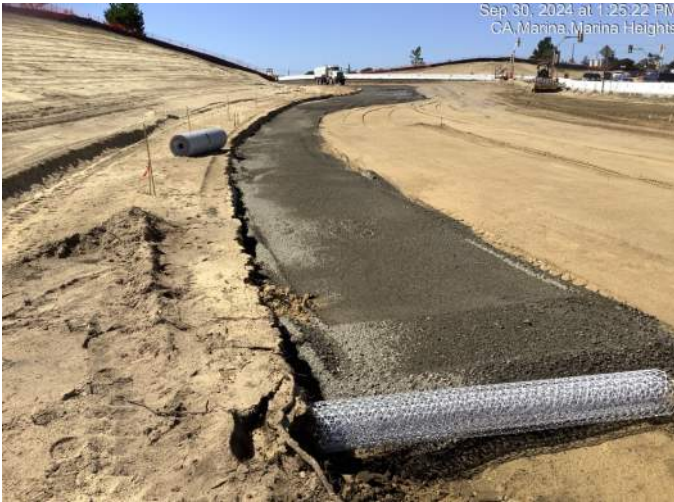
Geotextile material (roll in the foreground) is used beneath the base rock & asphalt to add strength to the roadway section.
