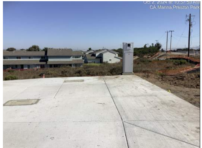
New power pedestal at Preston Drive. This will provide power to the street lights and irrigation controller.
