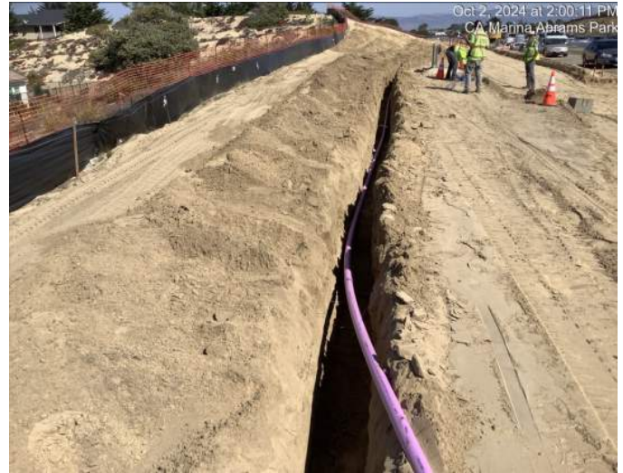
Installing irrigation service lines in trench between Abrams Drive and Marina Heights Drive
