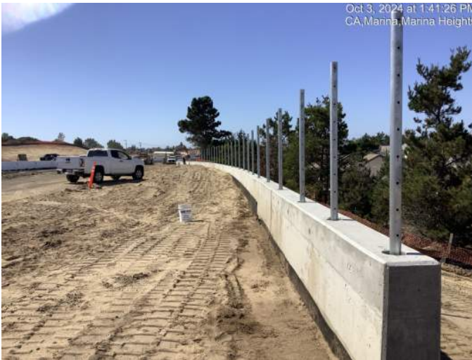
Installing posts on retaining wall near Abrams Drive. Installation of cables between the posts will follow.
