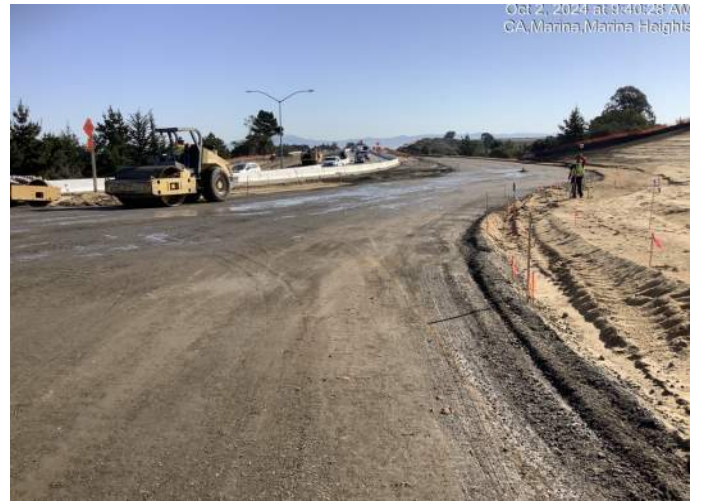
Compacting of base rock material. Contractor will do final grading and then pave the surface with asphalt.
