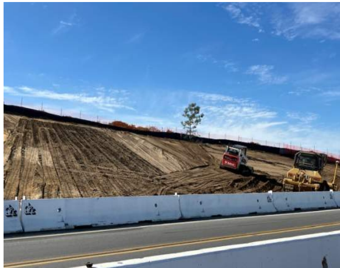
"Dressing" the slopes - equipment moves across the slopes providing final grading, compaction, and track marks that help hydroseeding take root.
