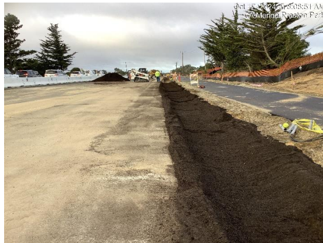
Installing Bio swale between new roadway and bike path, near Reservation Road
