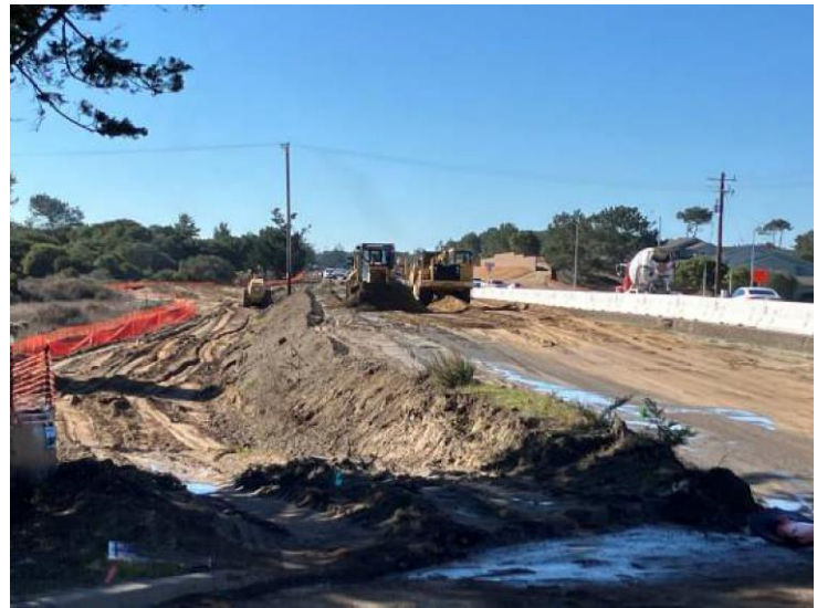
Earthwork to build embankment for a section of the widening between Preston Drive and Army Reserve driveway.
