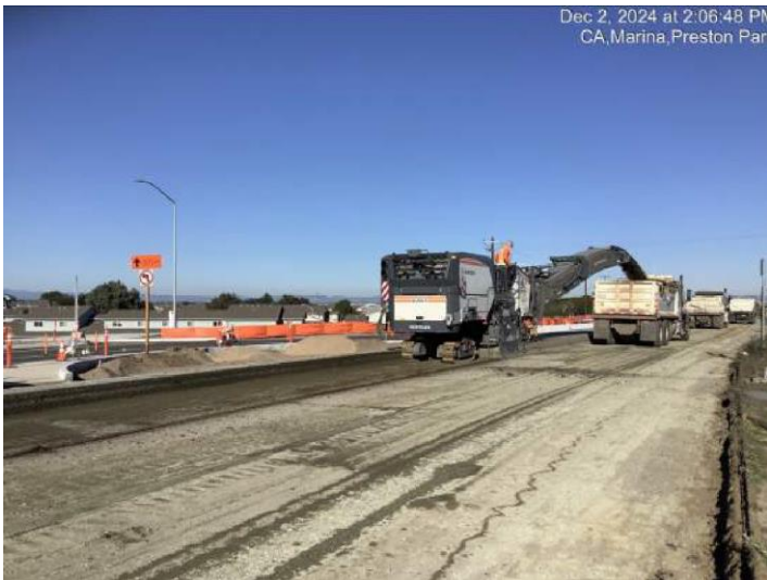
Grinding old pavement between Preston Drive and Army Reserve on south side of Imjin Parkway.
