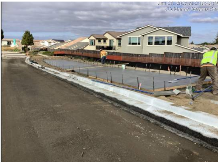
Curb & gutter previously placed. Crew finishing sidewalk concrete along Marina Heights Drive.
