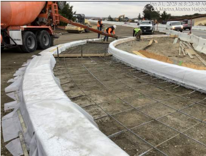
Placing concrete for truck apron portion of roundabout at Marina Heights Drive
