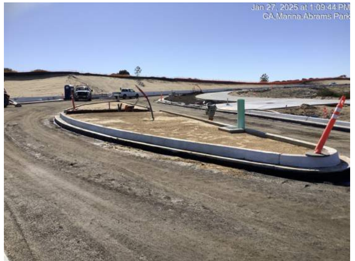
Curb & gutter, utility stub-outs, and median in-fill at the top of Marina Heights Drive
