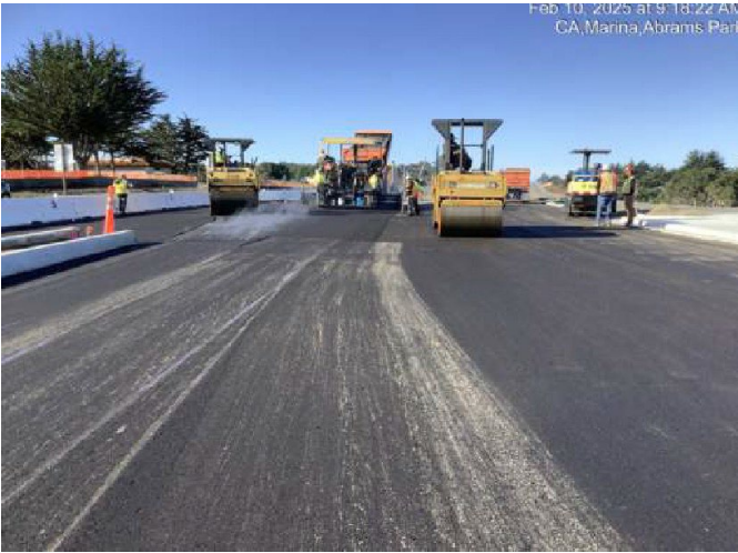
Paving first layer of asphalt for westbound lanes of Imjin Parkway (between Marina Heights Drive and western job limit)
