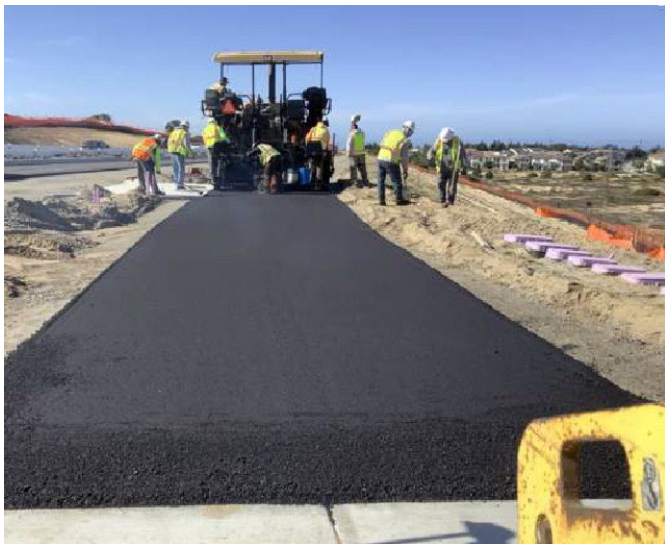
Paving bike and pedestrian path (between Marina Heights Drive and western job limit)
