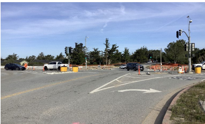
Abrams South side between Imjin Parkway to Bunker Hill will remain open and connected ONLY to Imjin Parkway with a signal, starting 3/26/2025
