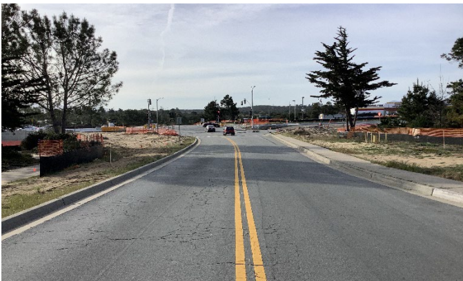
Abrams North side between Imjin Parkway to Brostrom will be closed for construction starting 3/26/2025
